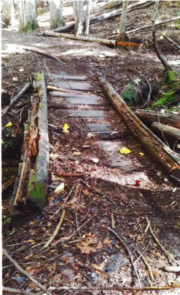
12' Bridge, 9/20/16. Deck is worn and broken, but substructure is relatively solid.
