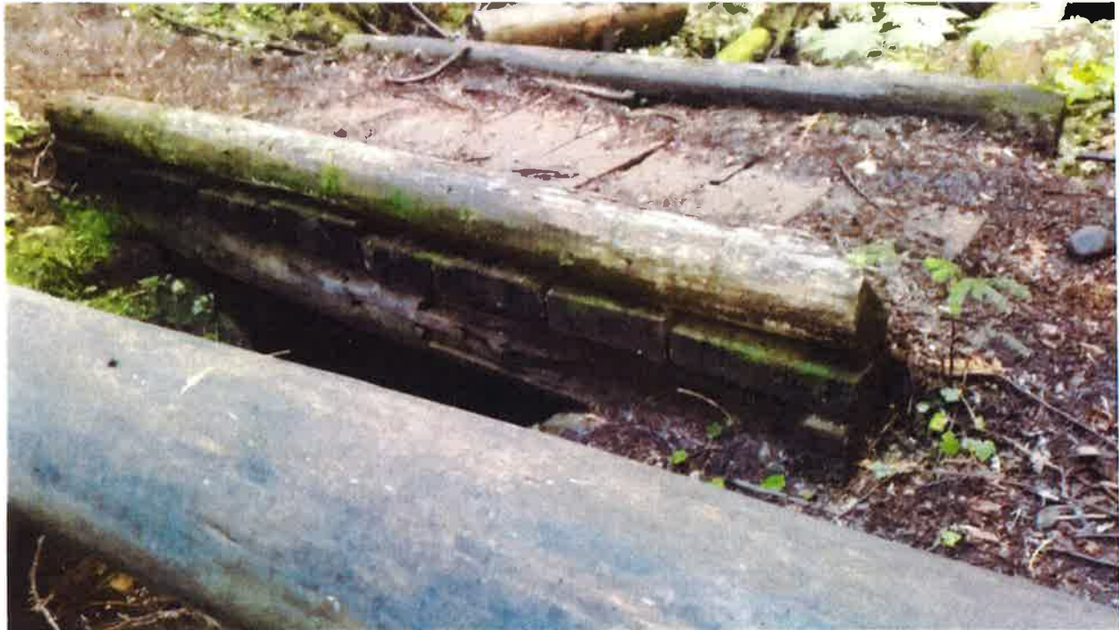
8' Bridge, 9/20/16. Notice the stringer in contact with the ground. It should be placed on a larger mudsill to prevent premature decay.
